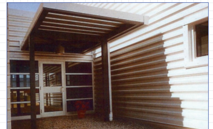
Icynene® insulation and air barrier system was installed because it contributes to the achievement of LEED credits, such as energy performance and thermal comfort.
