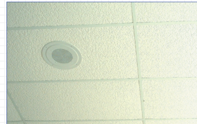
One year after the Icynene® insulation had been installed above these ceiling tiles – no more water damage.
