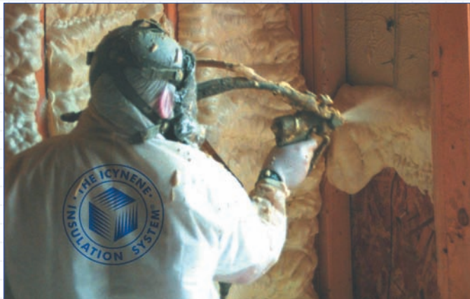
Icynene® is sprayed directly into the exterior wall. The foam softly expands to fill all of the cracks and crevices. Any excess foam is easily trimmed in preparation for drywall.
