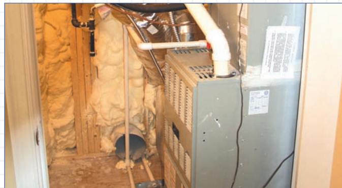
Icynene® was sprayed directly into the wall cavity around the HVAC system and the return and supply ducts. This helped to improve the airtightness of the building envelope and increase the overall energy efficiency.
