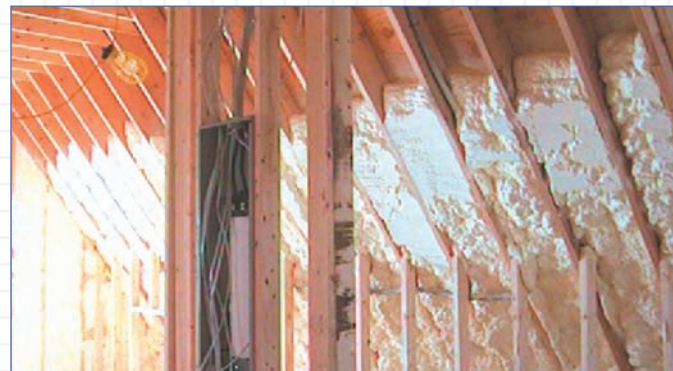
Icynene® was applied to the underside of the vaulted ceiling in the old attic space. This turned the previously unconditioned space into a conditioned living area.
