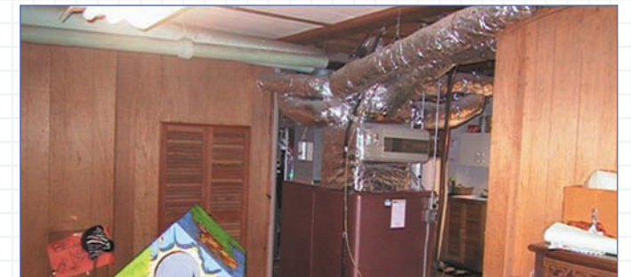
The original furnace and duct work in the house were circa 1970's. The air infiltration rate was 0.65 ACH (Air Changes per Hour) @ natural pressure. The Icynene® application reduced the rate to 0.37 ACH nat .
