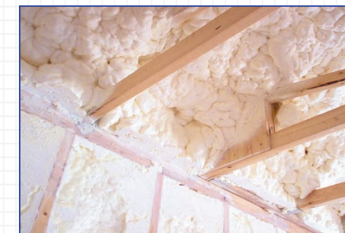
Icynene® softly expands to 100 times its initial volume to completely fill all gaps and crevices that compromise airtightness. Areas that are considered difficult to insulate with conventional insulations are no obstacle for Icynene®. Attics, ceilings, and walls can be quickly and easily insulated.
