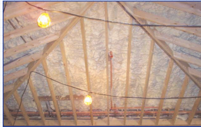
Icynene® was sprayed into the cantilevered overhangs and roof assembly to prevent warm, moist air from coming into contact with cooler surfaces, minimizing the potential for condensation.
