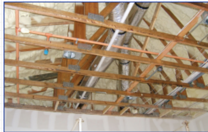
Icynene® was applied to the underside of the roof deck creating a sealed, unvented, and conditioned space for ductwork and air handlers. Photo courtesy of IBACOS, Inc. (www.ibacos.com)
