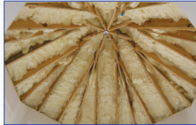
Icynene® soft foam insulation was carefully installed in the top of the two-storey entrance tower to minimize air movement and to insulate the home. Photo courtesy of IBACOS, Inc. (www.ibacos.com)
