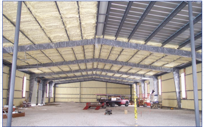
Once Icynene® was applied to the steel wall panels, tests revealed that the PFI building achieved an airtightness level better than that of a tight residential structure.
