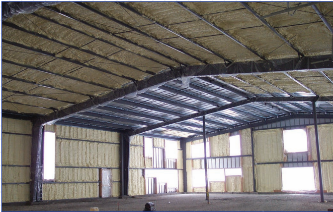
Icynene® soft foam insulation was sprayed at an average depth of 4-5 inches onto steel wall panels, gable ends and the underside of the steel roof.
